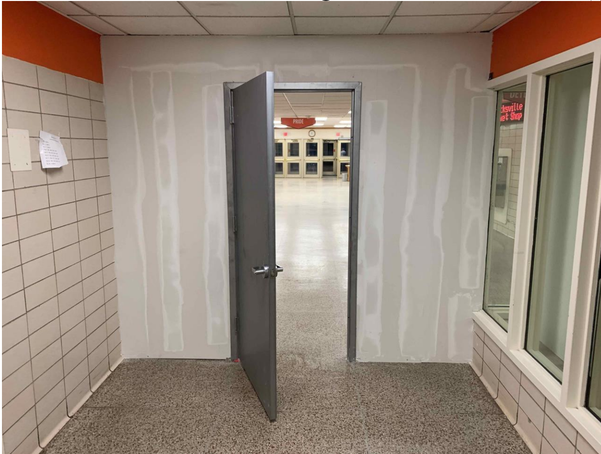
Temporary door and wall installed to mitigate dust and reduce unwanted foot traffic.
